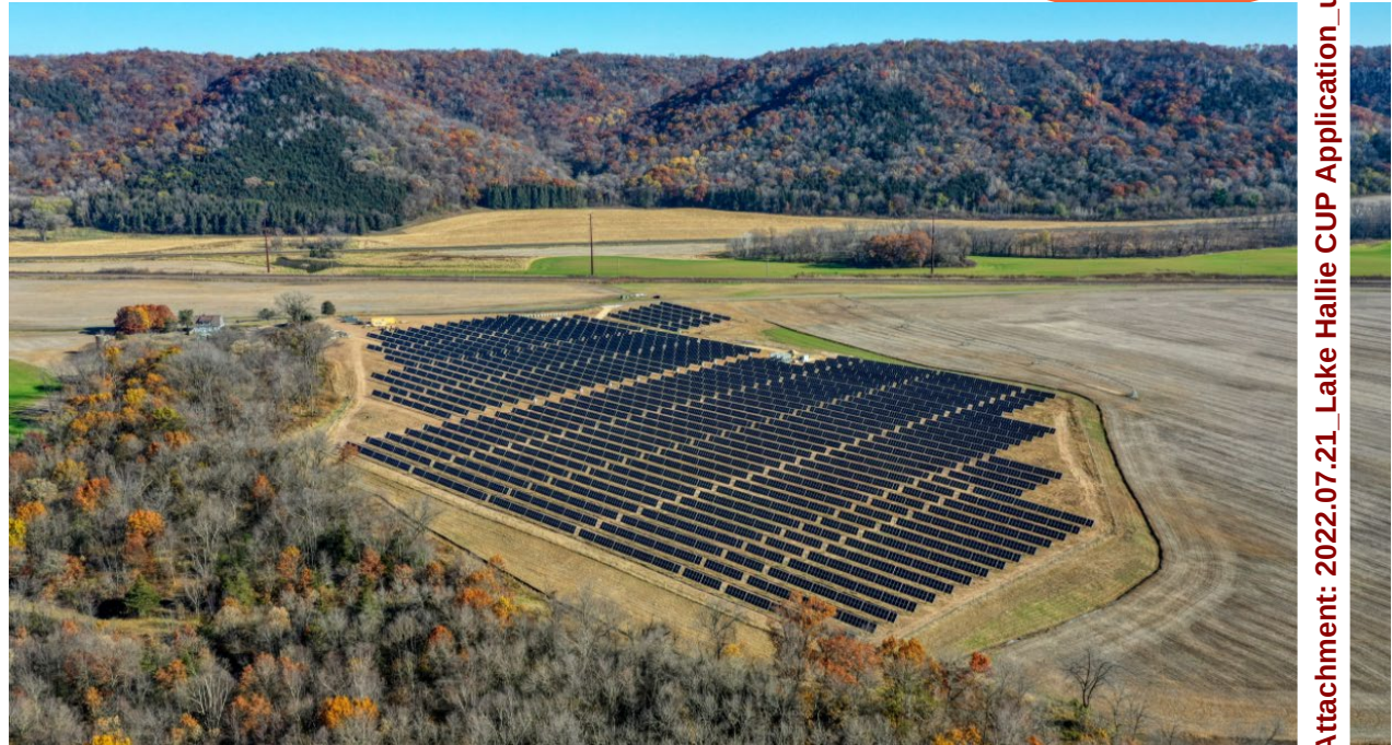
3MW Stromland Solar Project, Cochrane, WI
